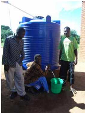
Water harvester installed at Chitedze 2 School
